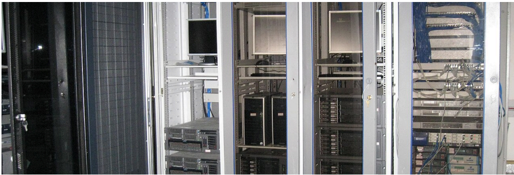
A server room run by Indian Railways. INDRAJIT DAS / CC BY-SA 3.0
